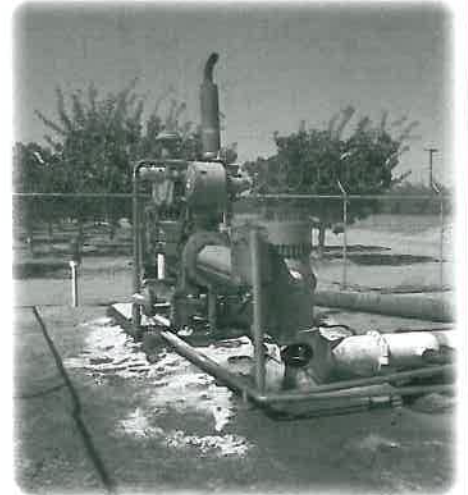
CCID HAS STEPPED UP GROUNDWATER MONITORING AND STUDIES IN LIGHT OF INCREASED PUMPING IN AND AROUND THE DISTRICT.
