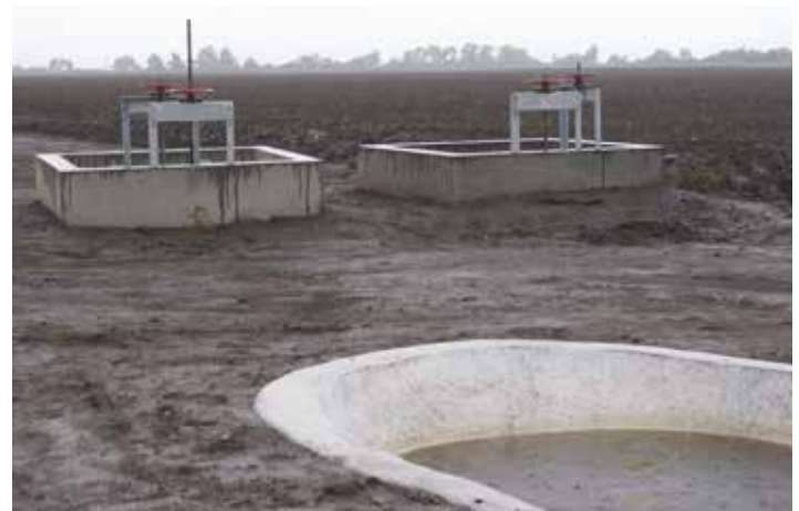
NEW WASHOUT DRAINS HAVE ELIMINATED MESSY WASHOUTS ON THE GAMBONI DITCH AND HELPED CLEAN UP FIELDS.
