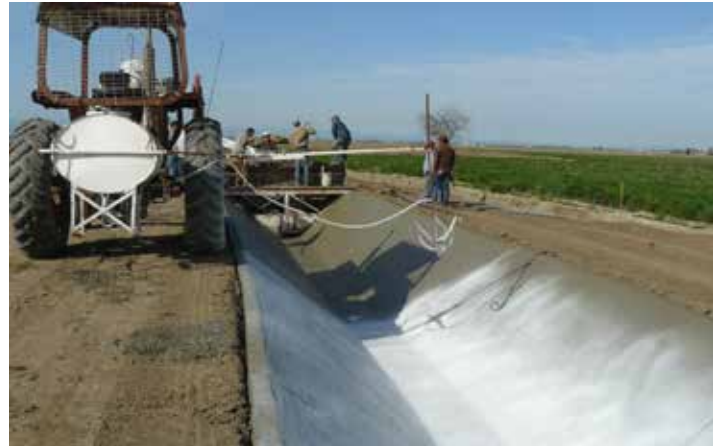
WORK ON THE SILO DITCH COMMUNITY DITCH IMPROVEMENT PROJECT INCLUDED REPLACING EARTHEN DITCH WITH MORE THAN TWO MILES OF CONCRETE LINING AND PIPELINE.
